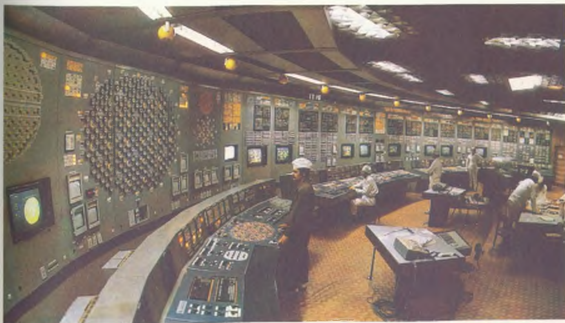
Ignalina Atomic Power Station: remote-control panel
